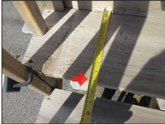
7. Stair run too small or not uniform
