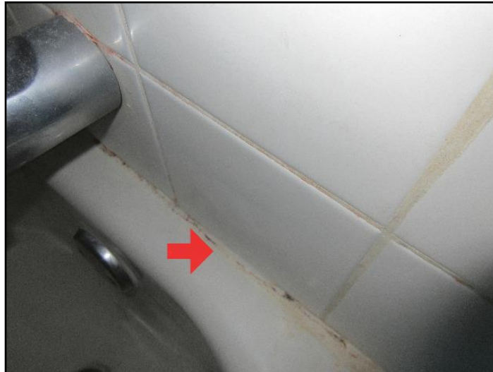
29. Caulking loose, missing or deteriorated
