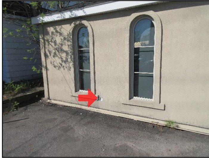
5. Mechanical damage, coach house
