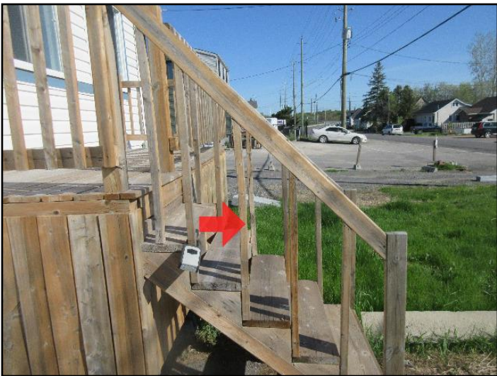
10. Openings too wide
