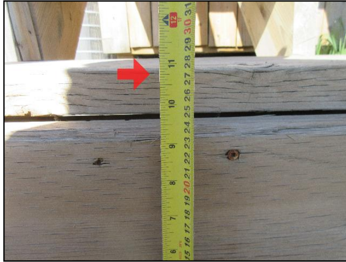
8. Stair rise too big or not uniform
