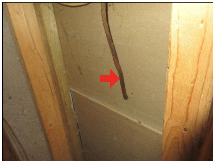
15. Not well secured
