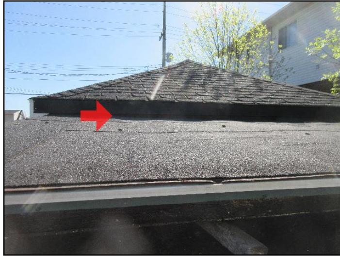
3. Damage, loose, open seams, patched
