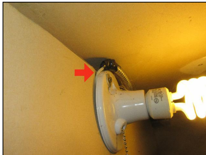
19. Wrong install (coach house)
