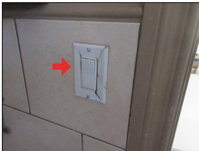
21. cover plate broken
