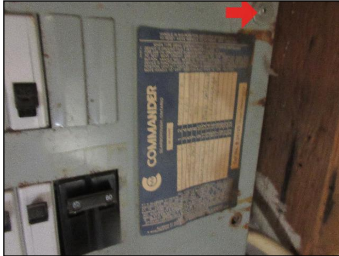
14. Inappropriate panel screws.
