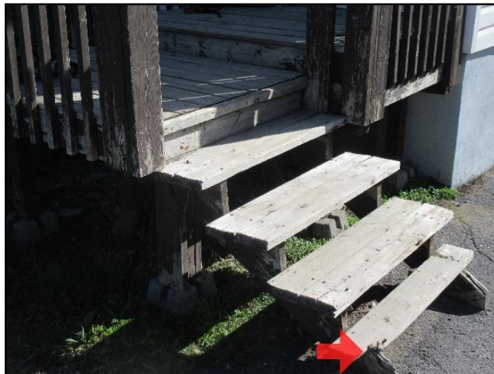
9. Stair rise too big or not uniform
